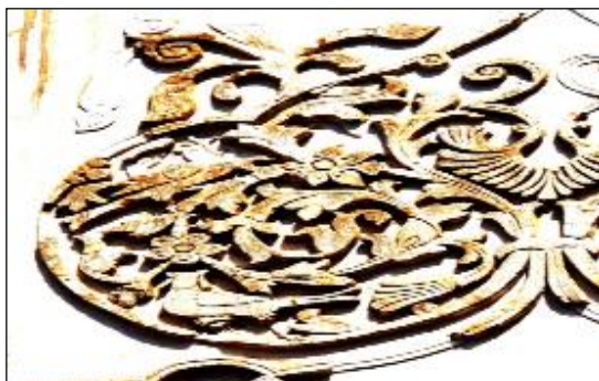
Figure 33: Bent lines in stuccos
