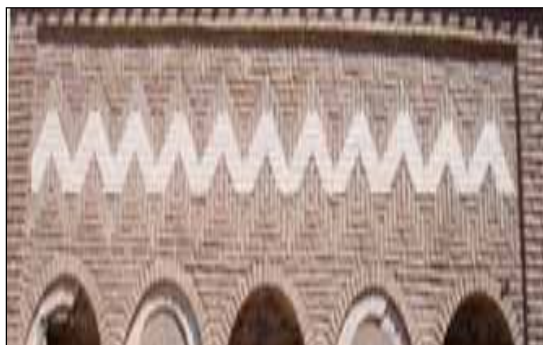
Figure 34: Zigzag lines in brick works
