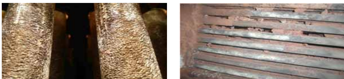
Figure 2. Corrosion and Suspended Particulate Matter on the Internal Pipes of the Heat Exchanger
