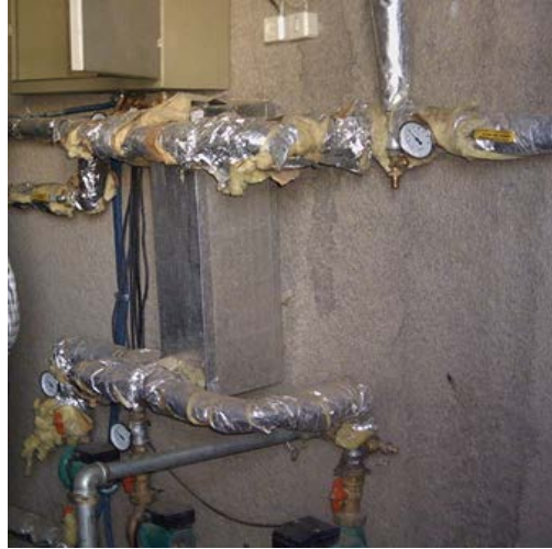
Figure 6. Plate heat exchanger and three circulation pumps
