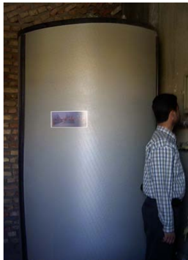
Figure 5. Wall steel tanks for water storage
