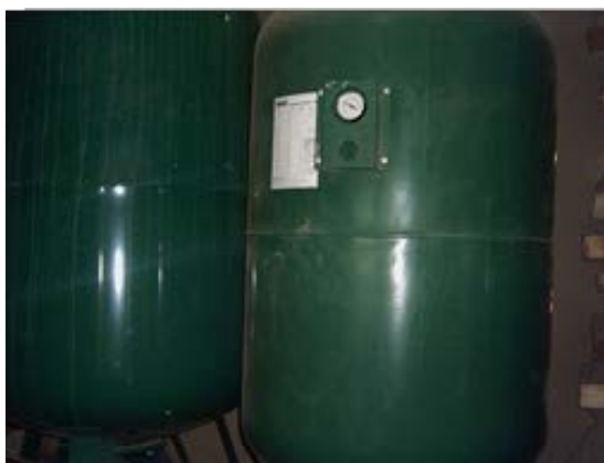
Figure 8. Closed expansion tanks
