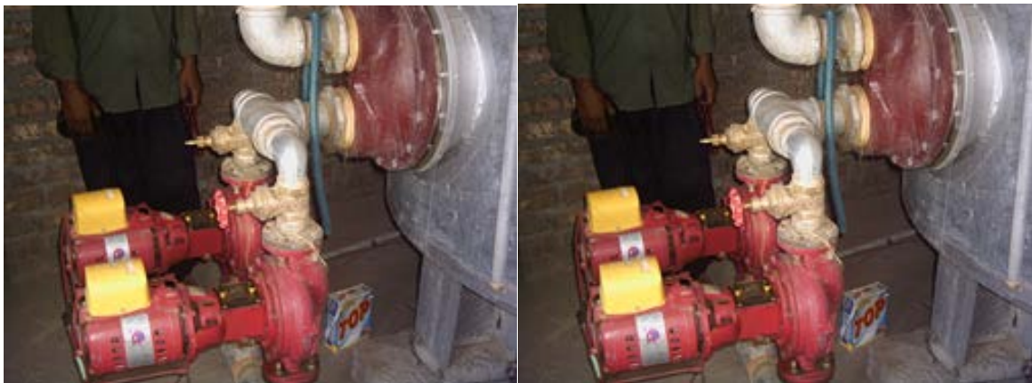
Figure 7. Coil of copper storage and two circulation pumps
