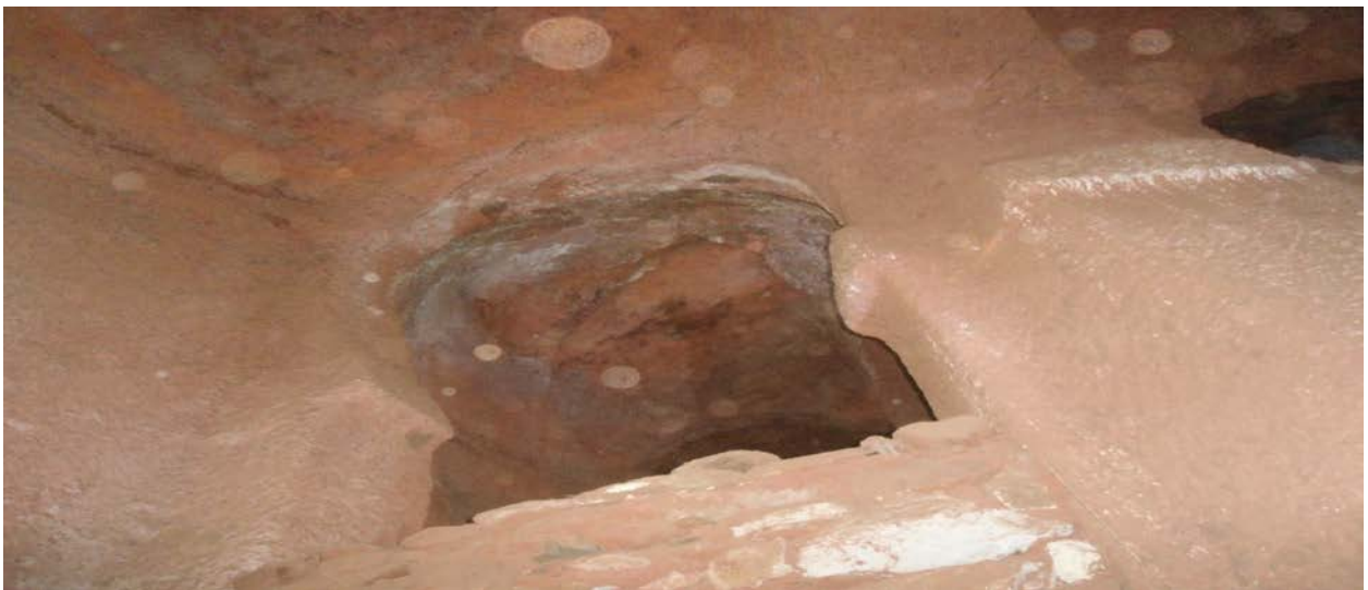
Figure 7 Seeing the damage to the interior walls and roof Source: by researcher (on March 24, 2020)
