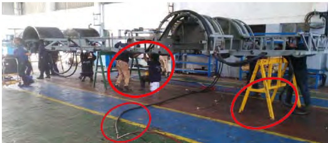
Figure 6. Shop floor workforces are assembling the Chassis standing on temporary benchwork (photo by authors)
